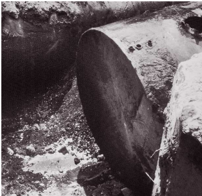
This tank excavation reveals a pool of leaked oil soaking into the ground.
