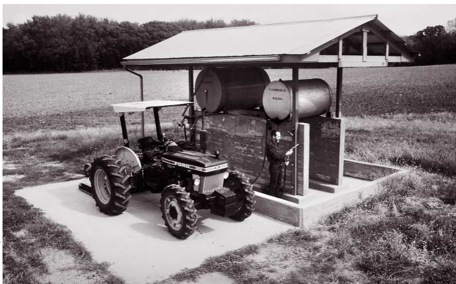
These above-ground tanks have a concrete pad and dike to contain spills and overfills.
