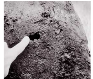
Old buried fuel tanks often rust through and leak contents directly into the soil.
